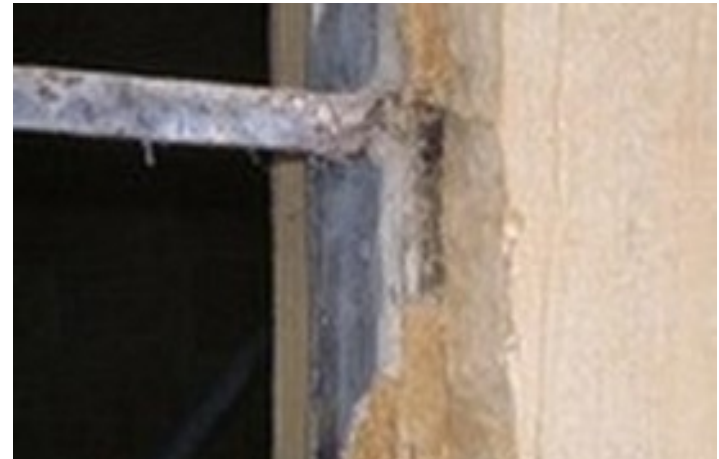
Corrosion of 16 windows' iron supports which expand to break surrounding masonry
